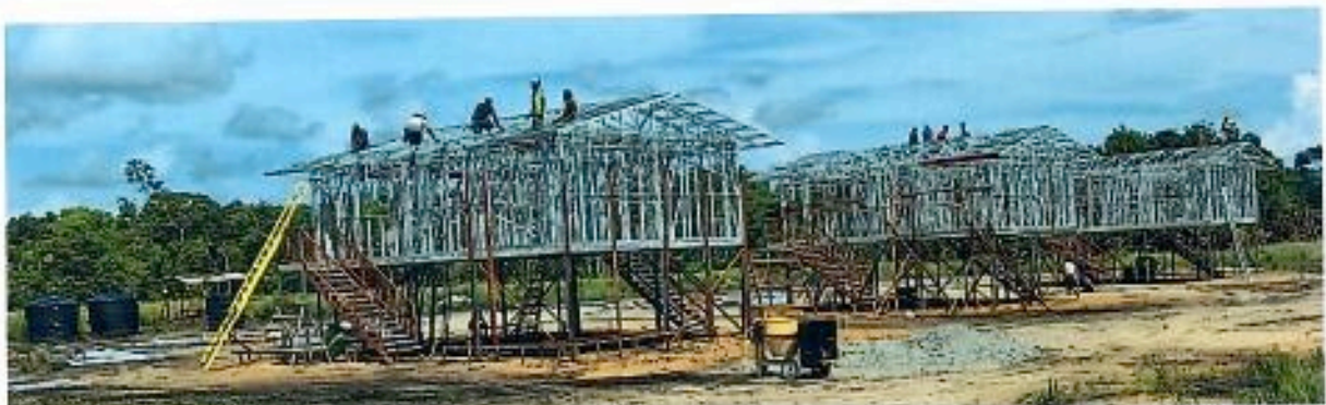
Three teachers houses' under construction at Edwaki High School in Telefomin District of West Sepik Province as part of the project obligations.
